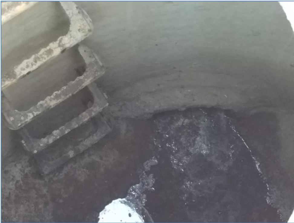
Figure 1: Sanitary Debris in the Palmer Street Inlet
